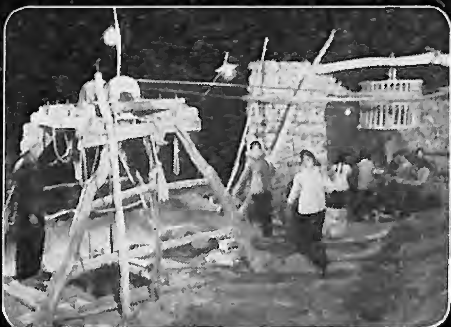
Work on the surface in cooperation with drilling the Dawn Tunnel below.
